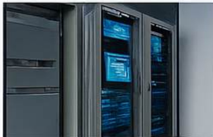
Station IT Rack / Ticketing
