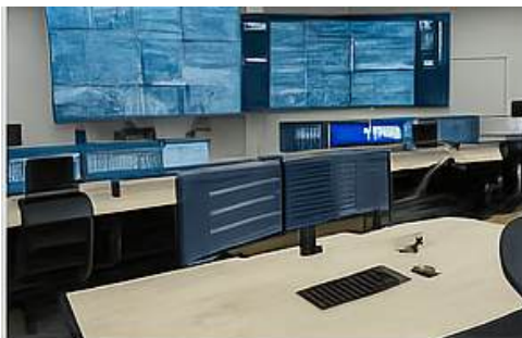
OCC Control Room
