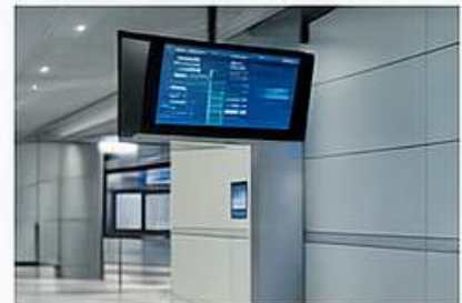
CCTV / PA / Passenger Information
