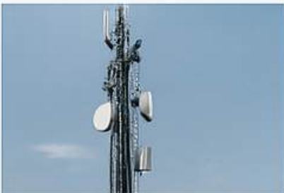
GSM-R / LTE-R Base Station
