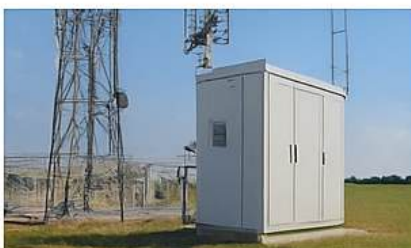
Telecom BTS Sites
