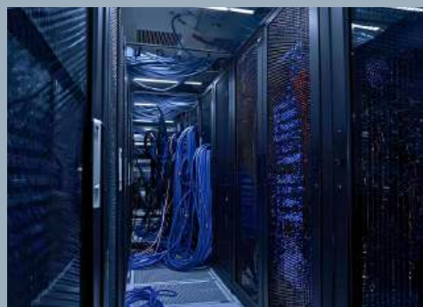
Enterprise IT Rooms
