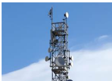
BTS Base Stations
