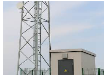
Radio Units & Base Stations
